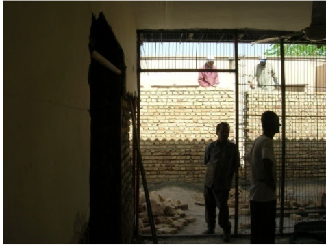
Fig. 18 Workers are demolishing some parts of an original PEH due to heterogeneity of local materials and those applied in original PEHs
