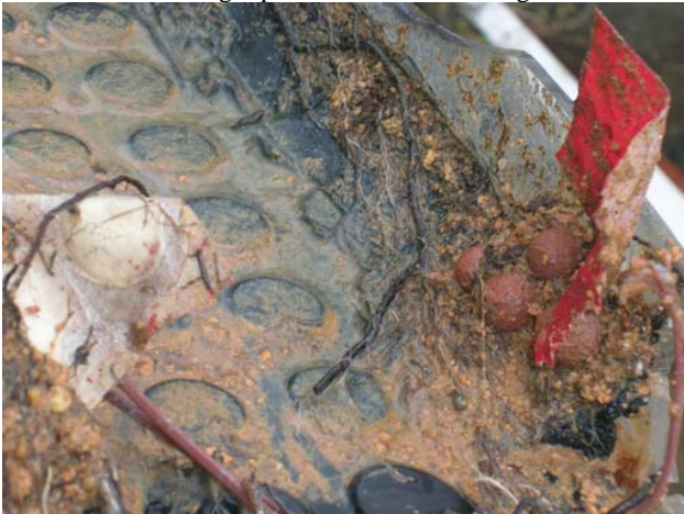
Fig. 6 Roots seemed to have grown into the liquid applied waterproofing at the edge
