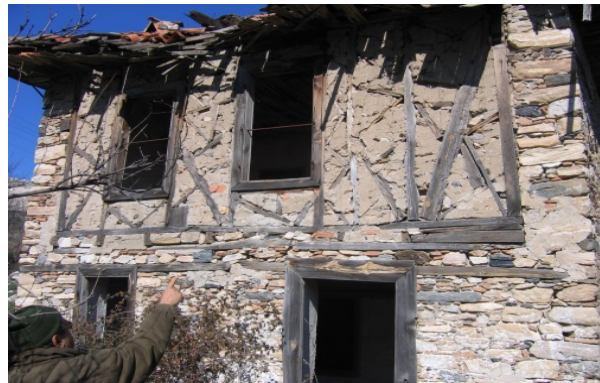
Fig. 3 A house abandoned by the effect of migration Eskişehir Village - Mugla
