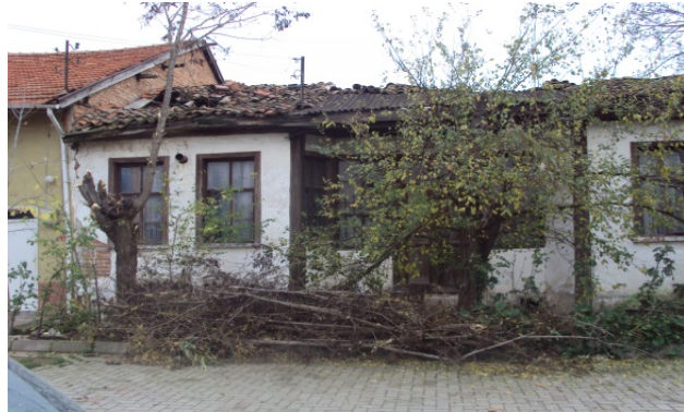
Fig. 2 A house about to collapse Karaagac – Edirne
