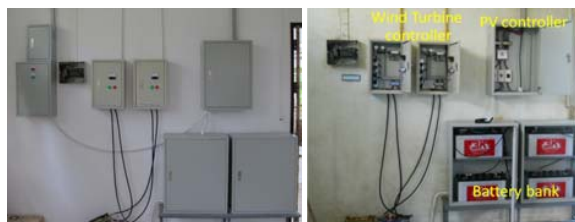
Fig. 4 The PV-Wind Charger and Controller and Battery Bank Installation
