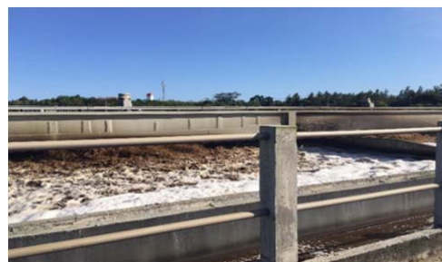
Fig. 1 Chemical effluent treatment station at CETREL
