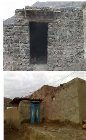
Fig. 1 A house with stone wall (left), A house with adobe wall (right)
