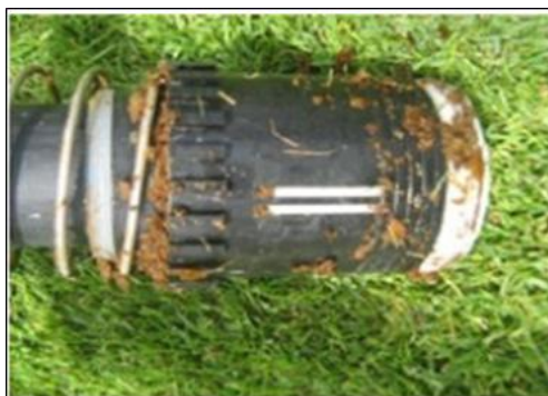
Fig. 2 Sprinkler clogged by scale
