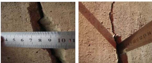
Fig. 5 5 Pier # 5 crack depth
