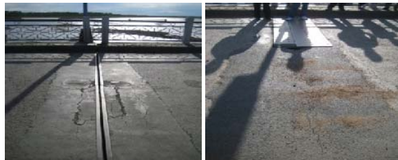
Fig. 11 Serious damaged bridge deck expansion joint
