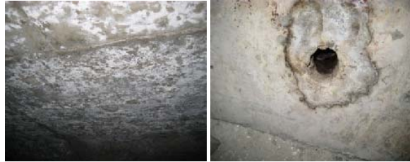
Fig. 9 (a) the internal box water drainage damage
