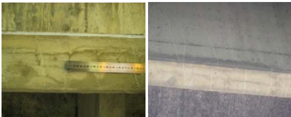
Fig. 9 (c) T beam cross-cracks in the region
