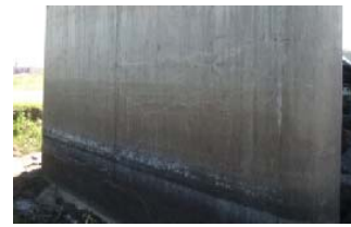
Fig. 7 Transverse cracks Pier #11
