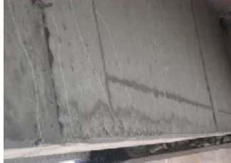
Fig. 9 (b) T beam cross-cracks in the region
