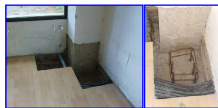
Fig. 16 Preparation of the anchorage zones of braces to the foot of a column
