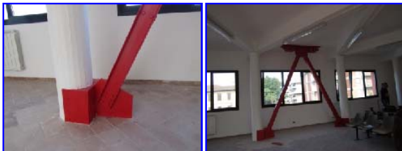
Fig. 18 Detail and general views of the other DB alignment parallel to x in the pilotis wing
