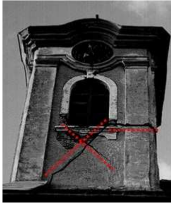
Fig. 15 Cracks at bell tower
