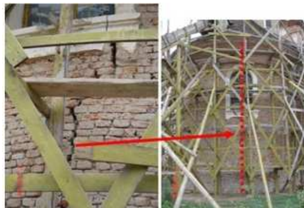
Fig. 14 Cracks at the eastern wall
