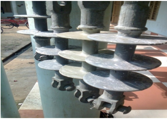
Fig. 5 11kV Specimen under urea pollution
