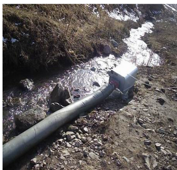
Fig. 4 Appearance of derivative micro HPP with pressure hose
