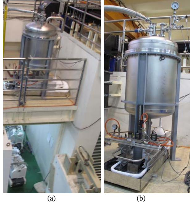
Fig. 4 Integrated with the passive and the flow control units, the buffer tank for vented nitrogen is located above the radiation-shielded area, in which the spare SRF module is cooled and tested
