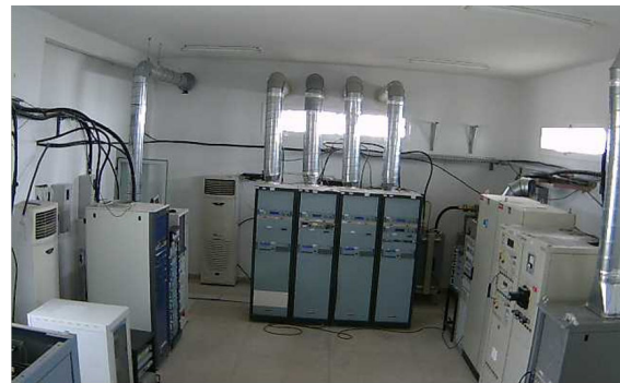
Fig. 2 The equipment's TV and radio FM broadcast centers (S7)
