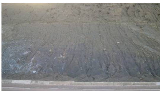
Fig. 4 Gully in road embankments in mudstones - Oued R'mel
