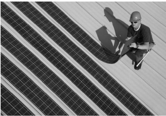
Fig. 8 Flexible solar panels for energy generation used in buildings
