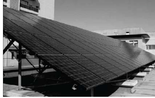
Fig. 2: The studied photovoltaic field installed in Tokyo University of Agriculture and Technology
