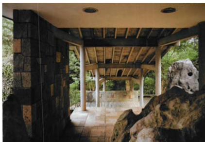
Fig. 4 The column-beam system of the roof and the multi-ribbed roof of the Xixi Scenery Spot Reception [3]
