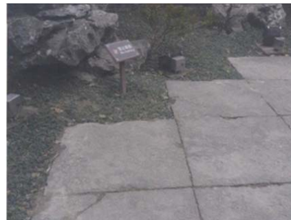
Fig. 12 The broken pavements in corners [10]
