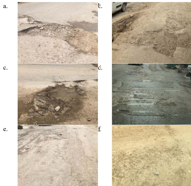
Fig. 1 Distress identified from Tripoli's roads (a. transverse crack, b. raveling (loss of coarse aggregates), c. potholes, d. bleeding and rutting, e. raveling and bleeding, f. fatigue/alligator cracks)
