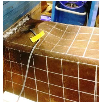
(a) Flange local buckling
