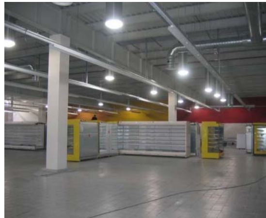
Fig. 3 Storeroom illuminated by light pipes
