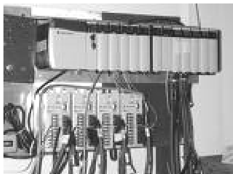
Fig. 2 A large PLC
