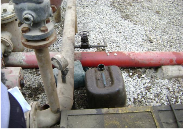
Fig. 10 Housekeeping of tank zone was found poor
