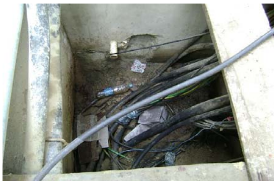
Fig. 14 Electric cable trench was found uncovered
