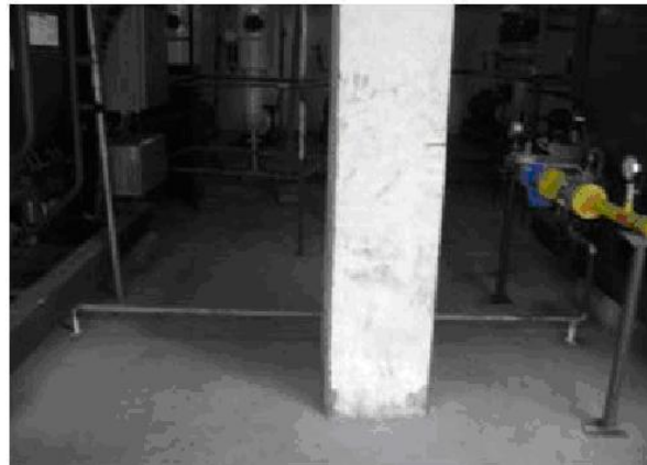
Fig. 11 Diesel dozing pipe has become a trip hazard
