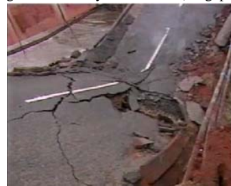
Fig. 2 Sudden collapse of Ynys-Y-Gwas bridge (UK, 1985)
