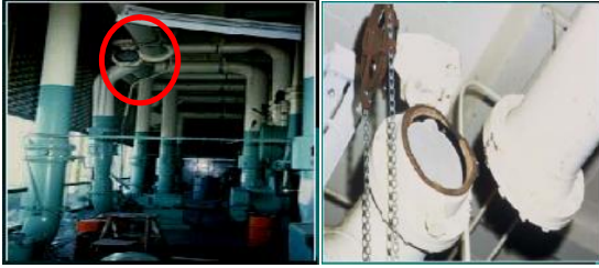
Fig. 1 Piping Failures in 1971 San Fernando Earthquake (Gates, 2005)
