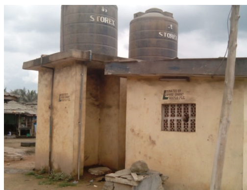
Fig. 6 Abandoned borehole due to contamination from Limestone
