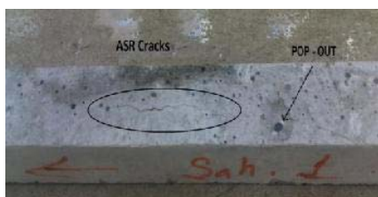
Fig. 5 Expansion cracking due to ASR and Pop-out of aggregate
