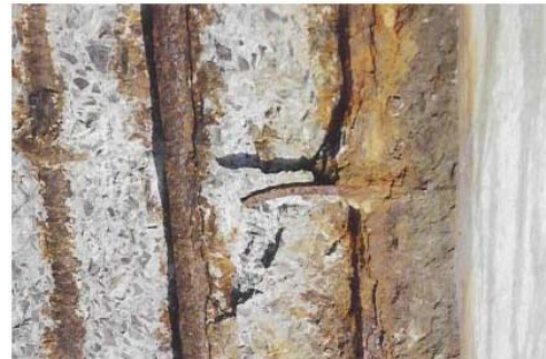
Fig. 1 Close-up of corroded rebars [5]
