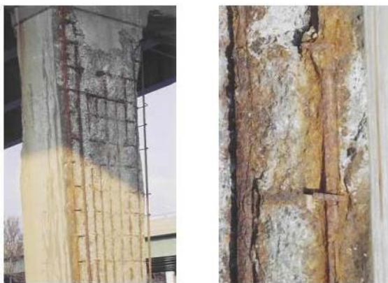
Fig. 3 Corrosion damage of tall concrete bridge pier columns [5]
