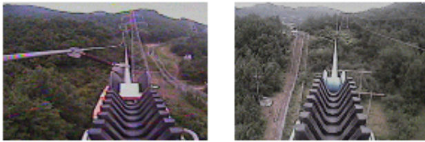
(a) Dual line test (b) Single line test Fig. 14 Actual line test on Sin-Okcheon Substation
