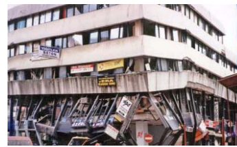
Fig. 1 A seriously damaged RC building in Marmara region [2]
