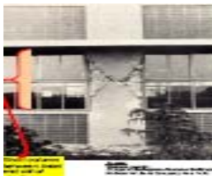
Fig.4. large window openings AND SHORT COLUMN
