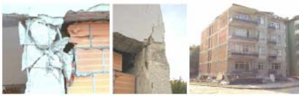
Fig. 9.Observed effects of interaction between infills and bare frame a)shear failure of column , b)exterior joint shear damage(Bonefro,Molise,2002) , c)global collapse for soft storey mechanism(Izmit,1999).
