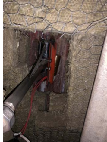
Fig. 5 Temperature sensor and heater installation
