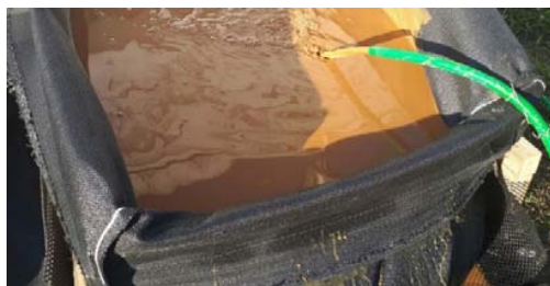
Fig. 2 Open geotextile system, drying bed
