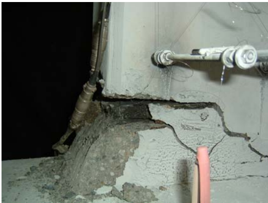
Fig. 3 Fallen state of the parts of the concrete at the upper corner of the corbel of the DP1R specimen
