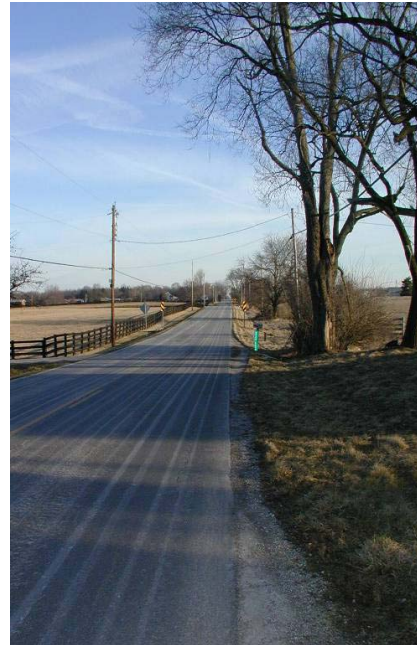
Fig.1 Failing Delaware County Pavement
