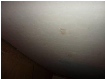
Fig. 2 Test slab after the 186 min of fire resistance testing – surface loaded by the high temperature
