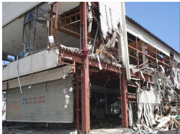
Fig. 12 Destruction of panels
