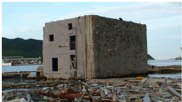
Fig. 22 Detail of slab foundation of collapsed building
