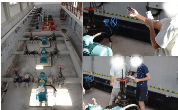
Fig. 5 Integrated pump house and pump test
