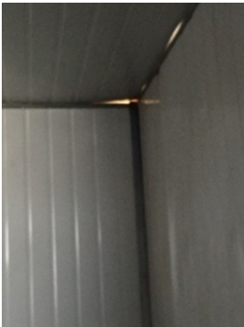
Fig. 5 Gaps between junctions [13]
