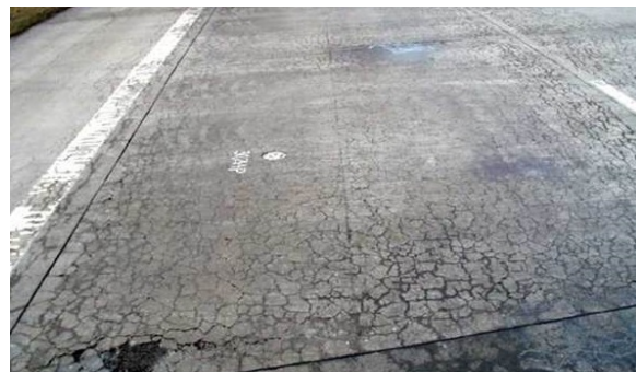
Fig. 1 Damage of top layer of the concrete road with RCA due to ASR
