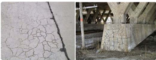
Fig. 4 ASR damage in highway projects [4]
