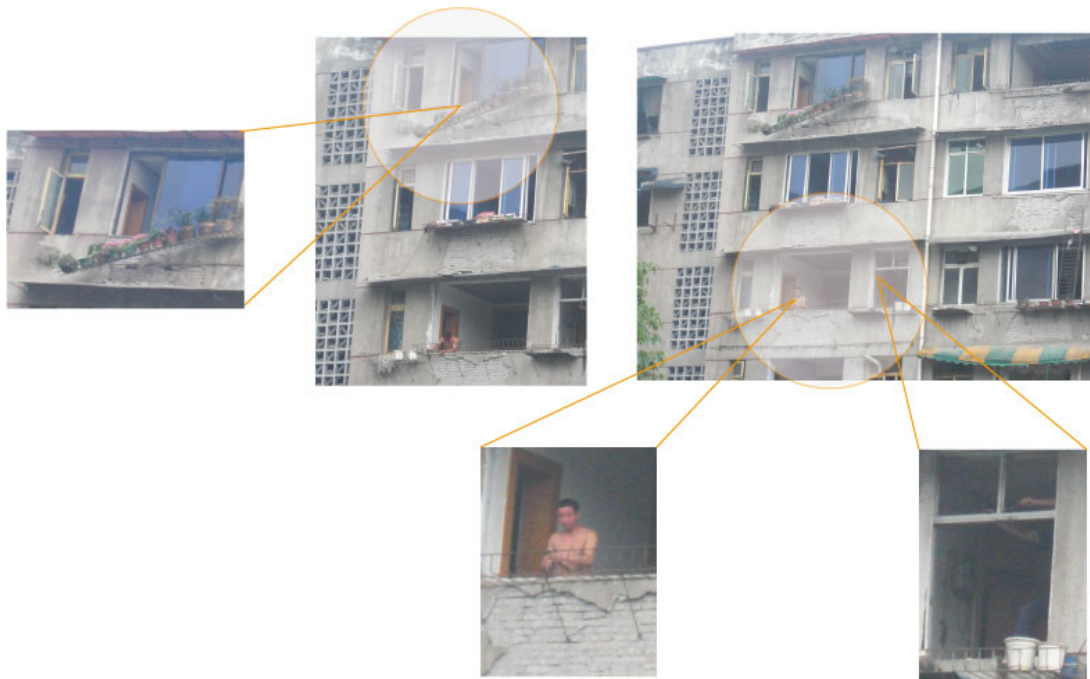
Photograph5. Danger posted by the Falling Objects
