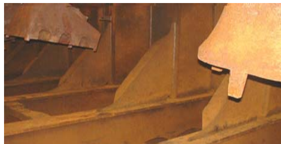
Fig. 1 Marine coating degradation showing rust in water ballast tanks [15]
