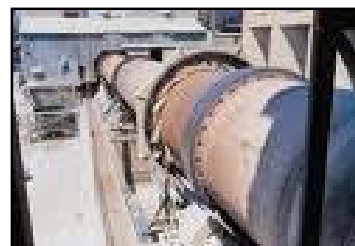
Fig. 1 Rotary Cement kiln
