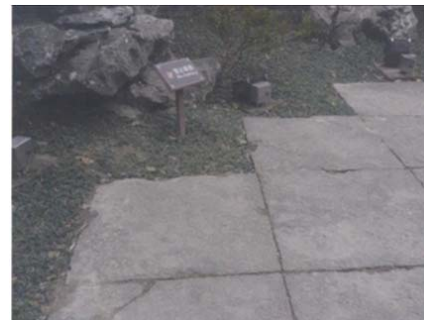
Fig. 12 The broken pavements in corners [10]
