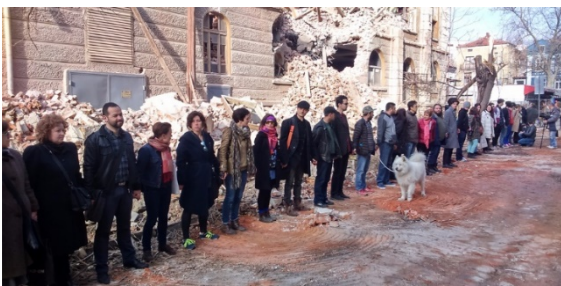
Fig. 6 The chain of citizens, trying to prevent the further demolition of the former warehouse [13]
