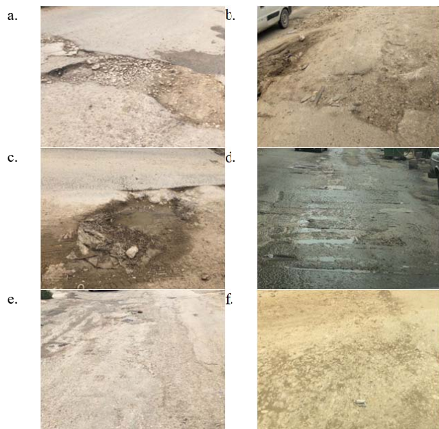
Fig. 1 Distress identified from Tripoli's roads (a. transverse crack, b. raveling (loss of coarse aggregates), c. potholes, d. bleeding and rutting, e. raveling and bleeding, f. fatigue/alligator cracks)
