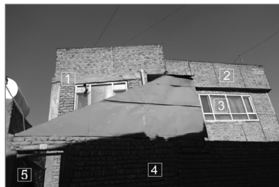
(c) A modern type of house: 1 – RCC roof, 2 – Fired-brick parapet, 3 – Wooden window, 4 – Fired-brick walls, 5 – Metallic main door
