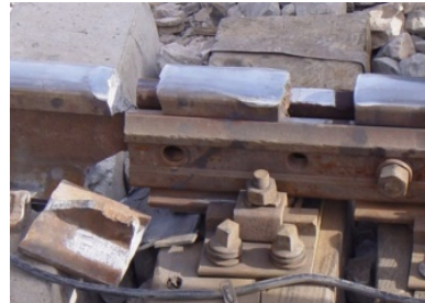
Fig. 1 Crack in rail bolt hole
