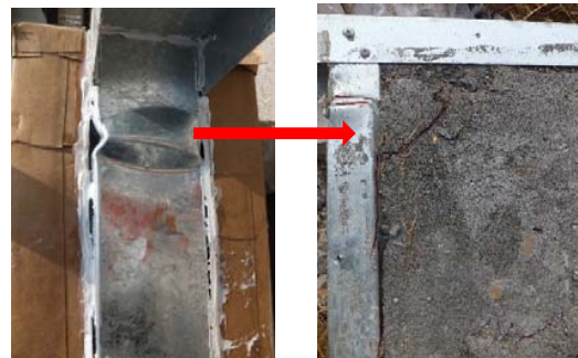
(c) Local buckling of W-3 CFS
