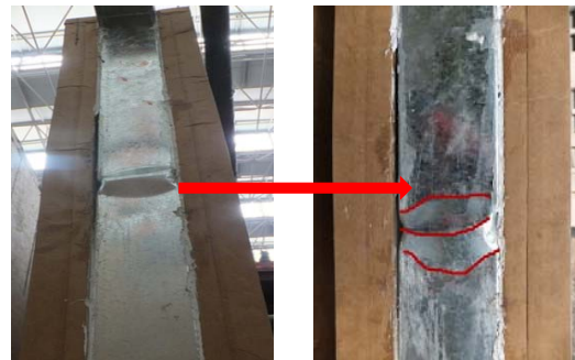
(b) Local buckling of W-2 CFS
